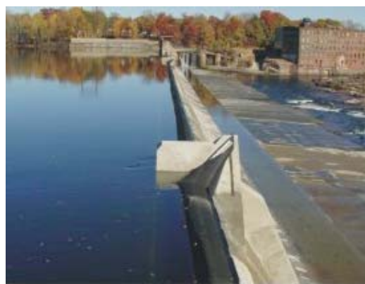
This dam on the Connecticut River is part of the Hadley Falls hydroelectric facility. Photo courtesy of HG&E.
