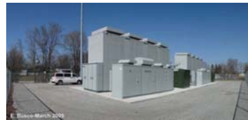
Sodium Sulfur Battery 2 MW
